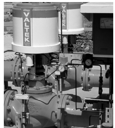
(right) A liquid nitrogen loading facility in Australia uses two Mark One valves for its emergency fire water system.
