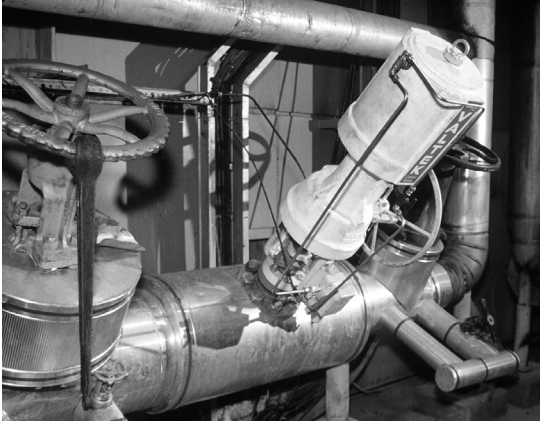
A 4-in Mark One with side-mounted handwheel operates a boiler feedwater system at a pulp plant.
